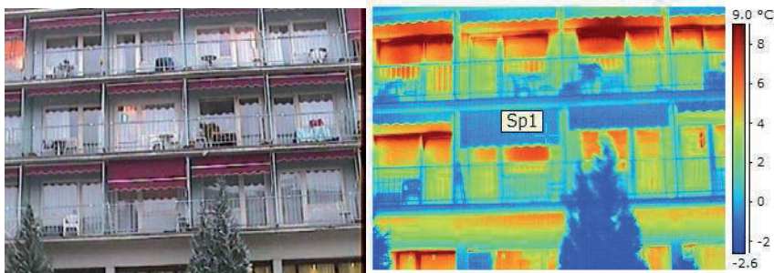
Illustration 5: Thermal losses through uninsulated cantilevered balcony slabs and windows
